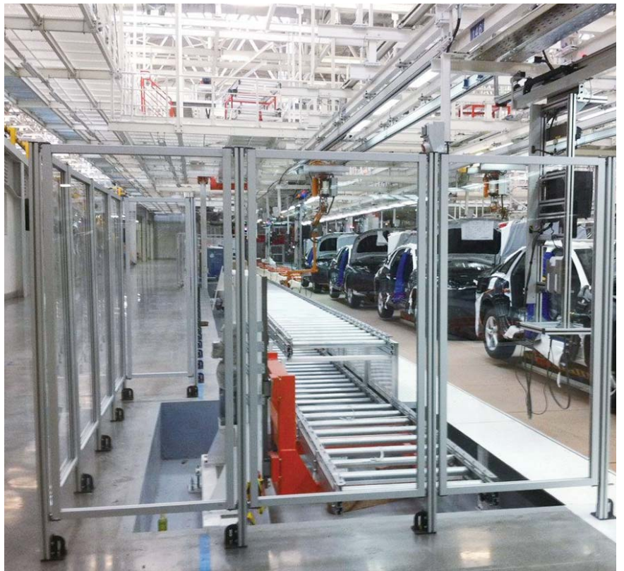
Protective barriers for car assembly line 汽车生产线外围防护
