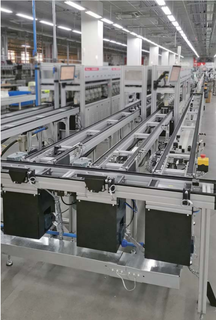
Pallet conveying control system 托盘输送控制系统
