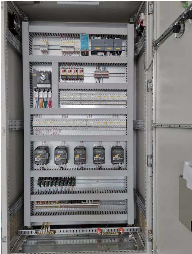
Electrical Control Cabinet 电控柜
