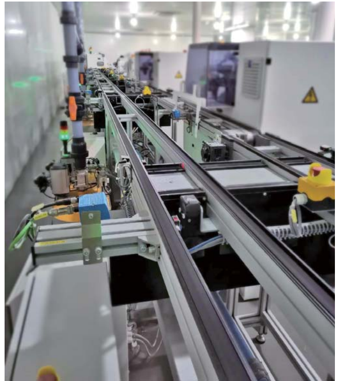
Pallet conveying control system 托盘输送控制系统
