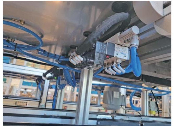
Solenoid valve and air pipe 电磁阀及气管
