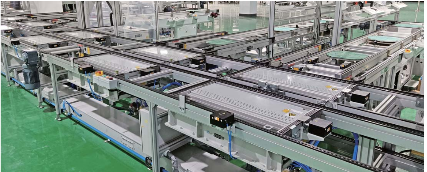
Pallet conveying control system 托盘输送控制系统
